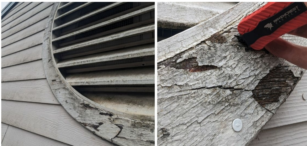
Figure 10. Station 93 Exterior Trim Dry Rot
