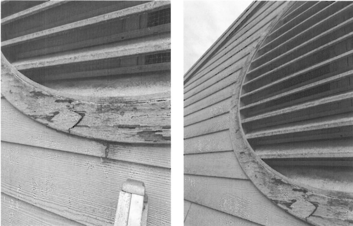
Figure 5. Trim Dry Rot at Station 93
