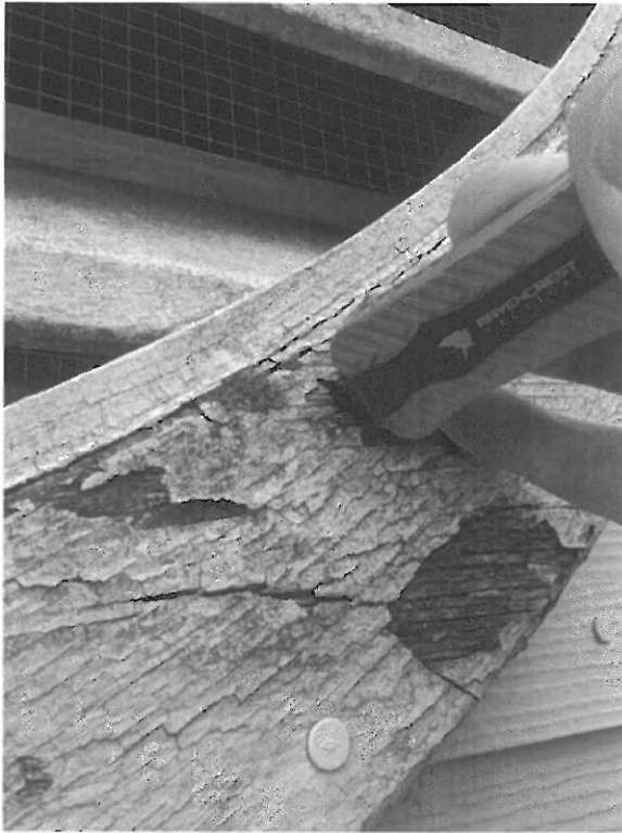
Figure 5. Trim Dry Rot at Station 93
