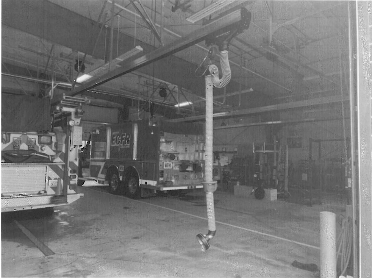
Figure 4. Station 91 Diesel Exhaust Extraction System
