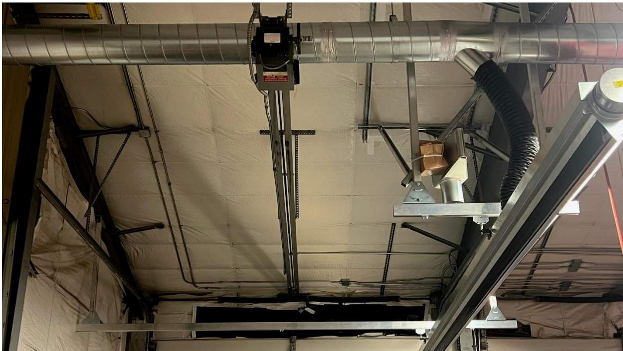
Figure 32. Inoperative Overhead Door Motor, Bay 4
